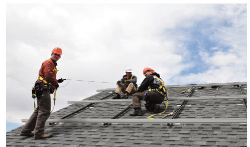
Rails/Racking Attached to the Standoffs
