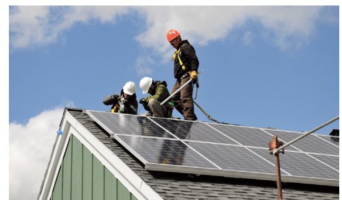
Modules Attached to the Racking
